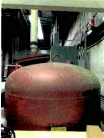
Photos Expansion tank 192623AK
